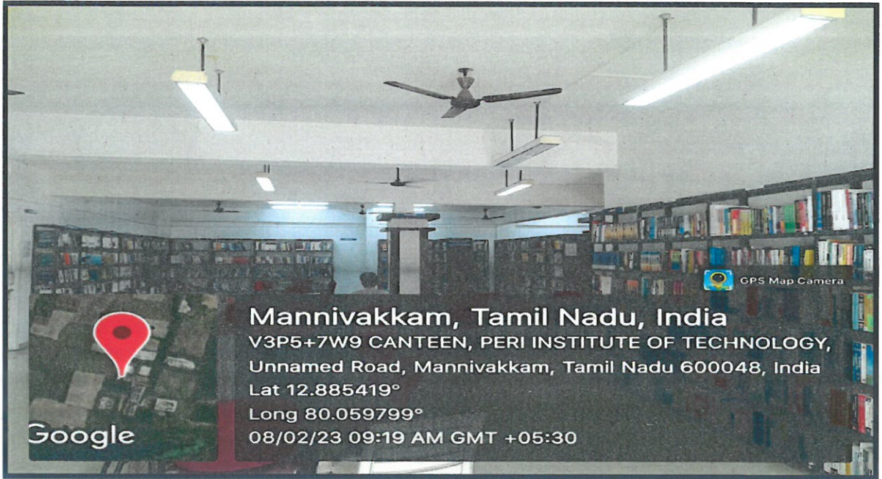
LED lights in "LIBRARY"
